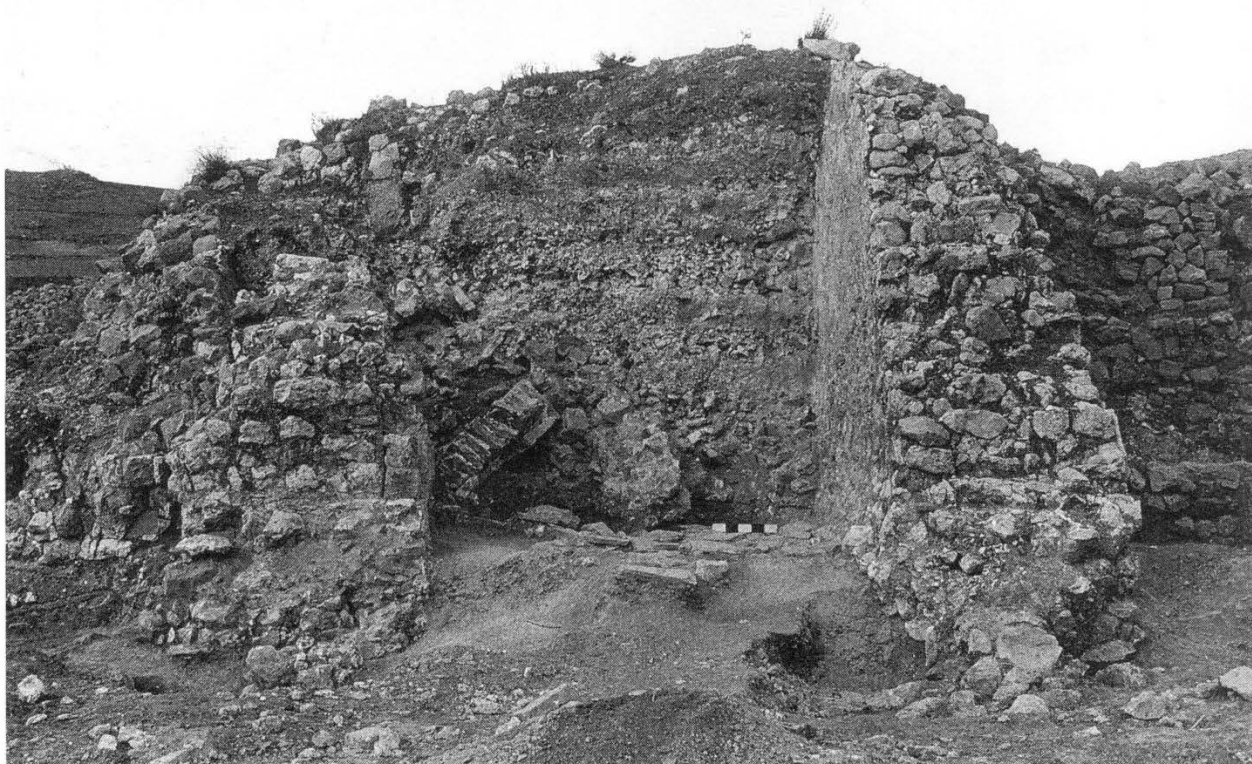
3. Building debris dumped on top of collapsed vault, Qal'eh-i Yazdigird.
