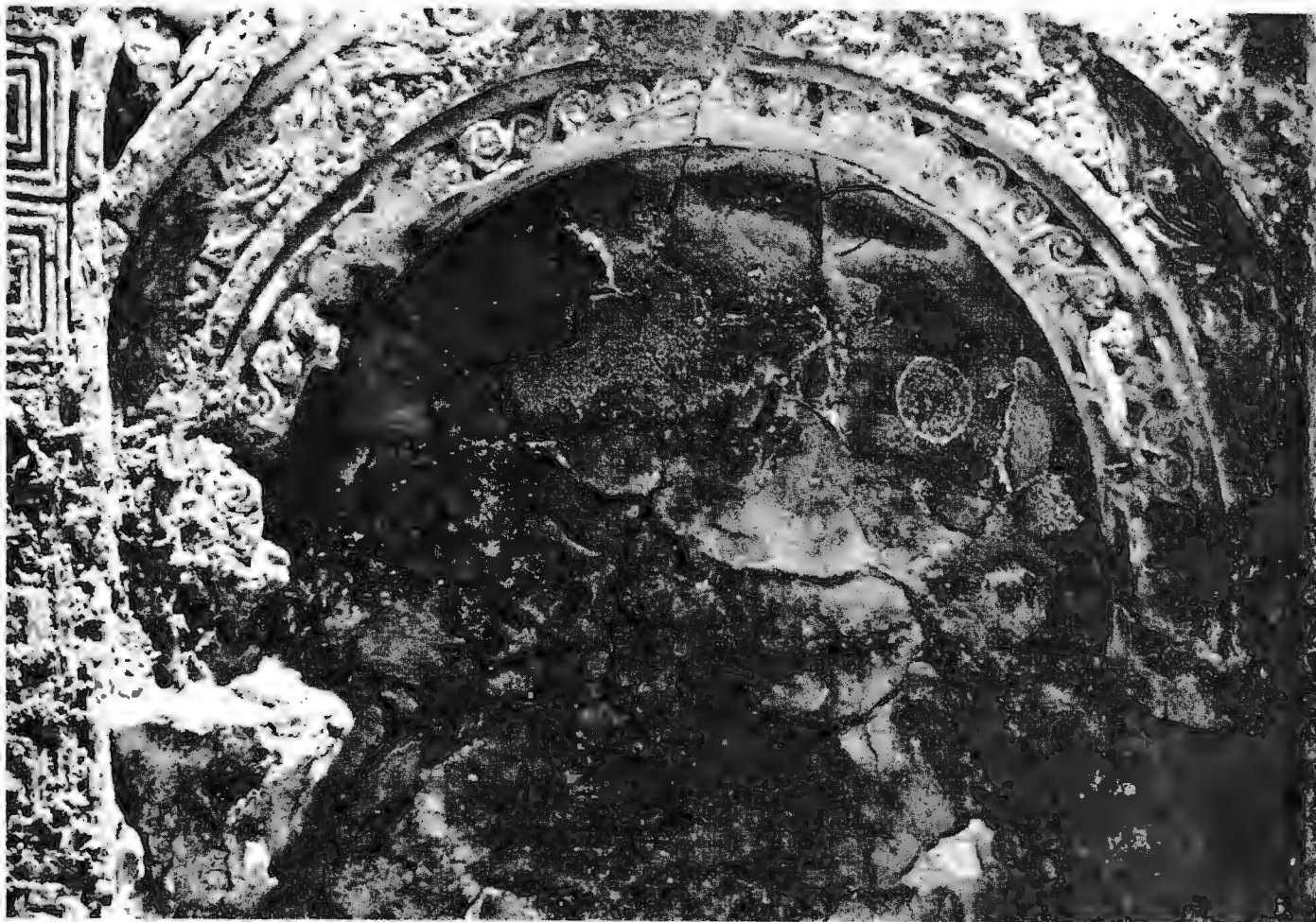
Pl. Va. Gach Gumbad, E2S2 Area 5. Niche 2 showing eroded edge of soffit.
